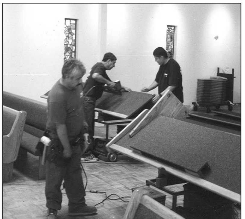
WORKERS LABOR - To install the new pews in preparation for a dedication service this weekend at Messiah Lutheran Church of Downey.
