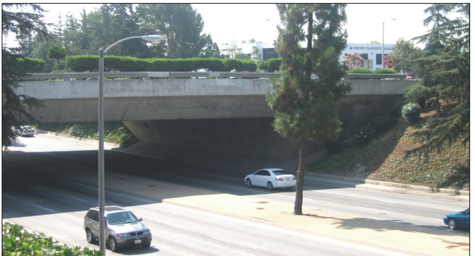
This bridge, spanning Imperial Highway between Rancho Los Amigos National Rehabilitation Center and Downey Municipal Court, garnered an 87.5 percent sufficiency rating, but was listed as "structurally deficient" because of "serious" deck concerns. Photo by Eric Pierce
