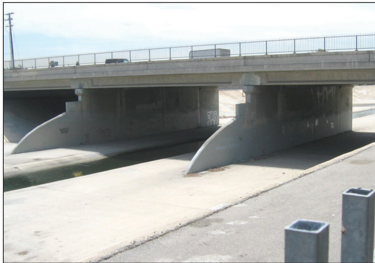
Three Downey bridges have been labeled "structurally deficient" by Caltrans and the Los Angeles County Department of Public Works, including the one above on Imperial Highway, crossing over the San Gabriel River. Officials, however, stressed that the bridges are safe. Photo by Eric Pierce
