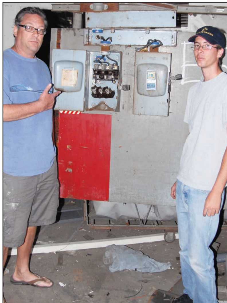
Gary DeRemer, left, and Andrew Malarkey stand next to where thieves pulled copper wiring on the south campus of Rancho Los Amigos National Rehabilitation Center. The theft has left the Downey Rose Float Association without the electricity needed to build a float. Photo by Art Montoya
