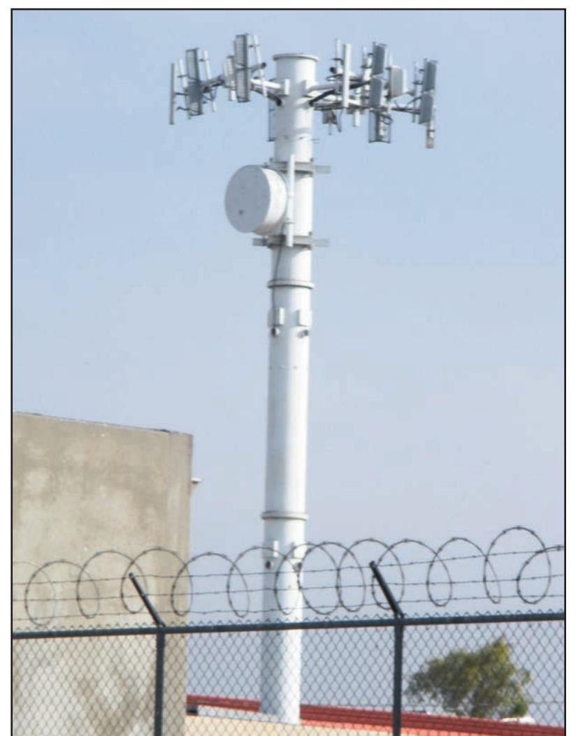
Monopoles, like the one pictured above at Firestone and Paramount boulevards, can be disguised to at least partially integrate into its surroundings, some more effectively than others. Photo by Eric Pierce
